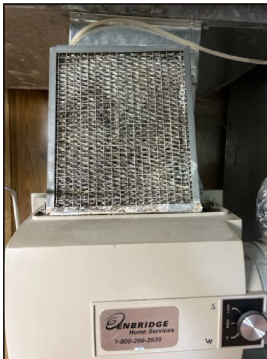
Mesh pad dirty/clogged
