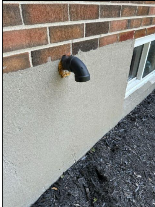
Vent termination problems
