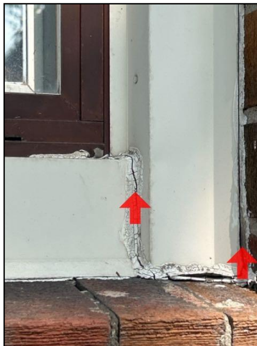
Caulking missing, loose or deteriorated
