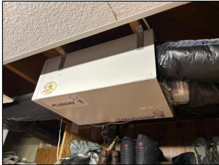
Passive air exchanger
