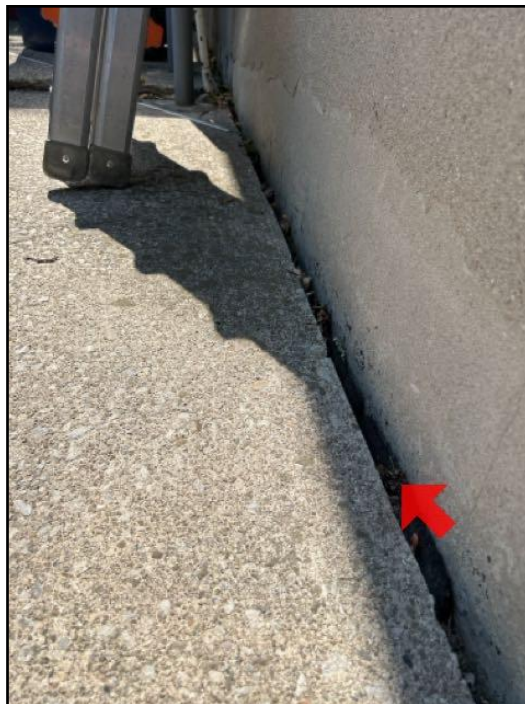
Unsealed gap at building
