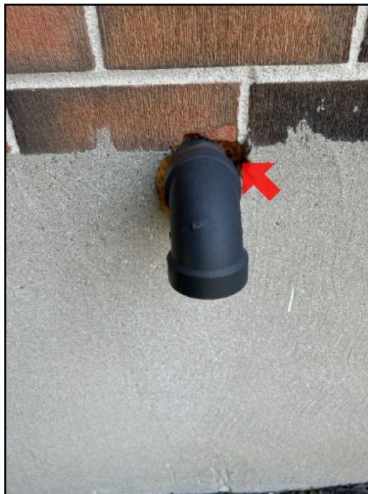
Caulking missing or ineffective
