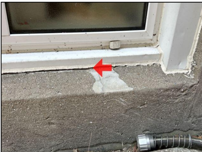
Caulking missing, loose or deteriorated
