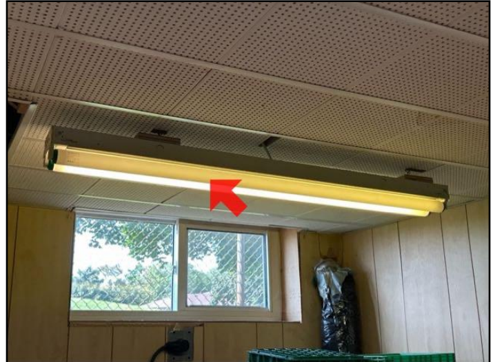
Exposed to mechanical damage (No cage or...
