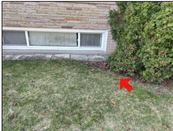
Improper slope or drainage
