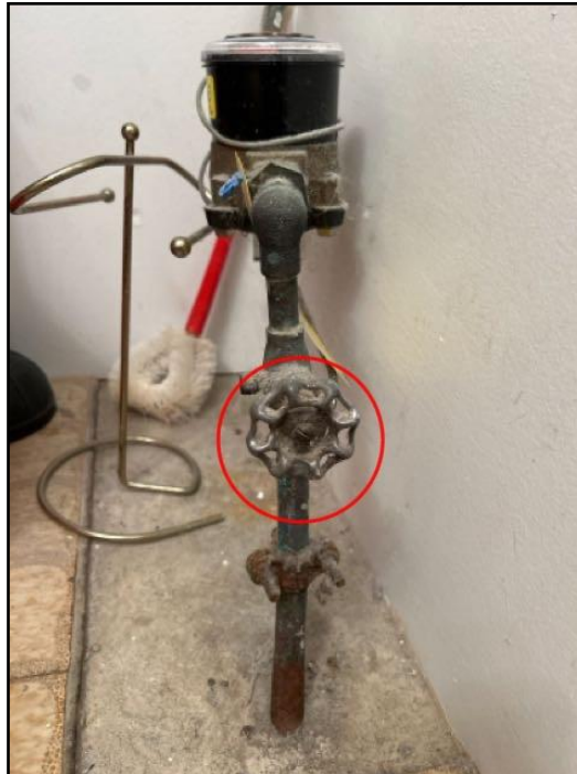
Water shut-off valve
