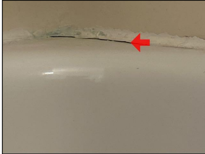
Caulking loose, missing or deteriorated
