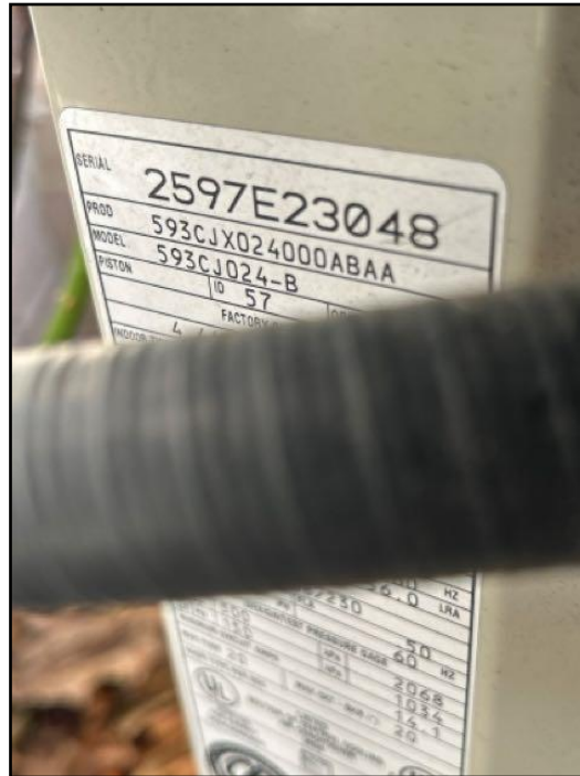
Air conditioner data plate
