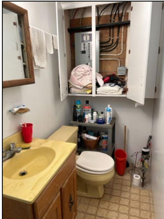
Poor location for panel
