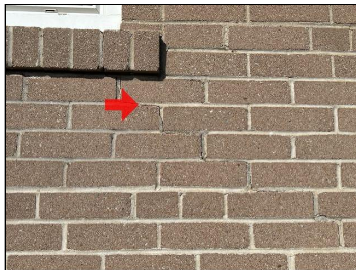
Typical minor cracks
