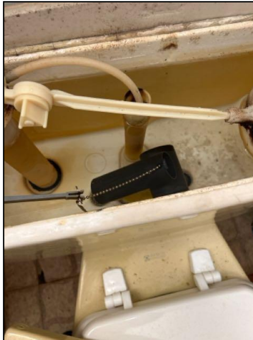
Obstructed or weak flush
