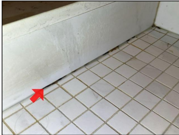
Caulking loose or deteriorated
