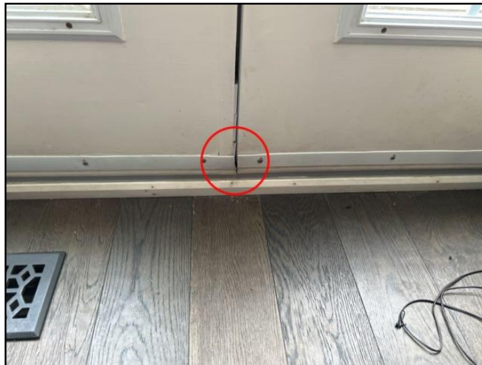
Weatherstripping missing or ineffective
