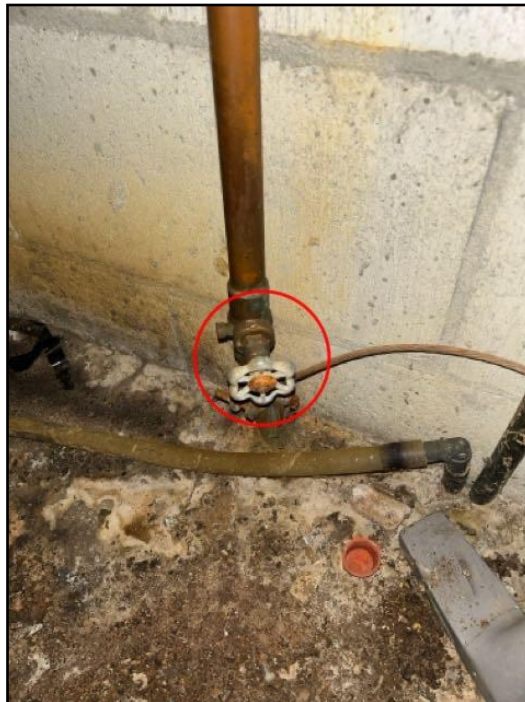
Water shut-off valve
