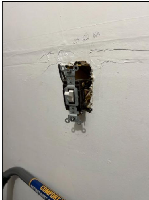
Loose, missing cover plate
